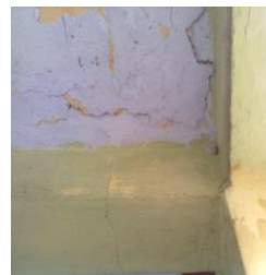
Figure.7. Beam and slabs were of in-situ concrete. Shear failure on floor at cement mortar
