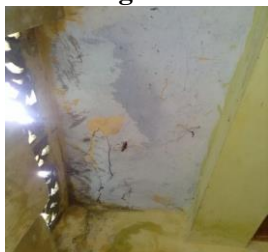
Figure.6. Floor bent with the beam but shear failure occurs. Fine crack on floor
